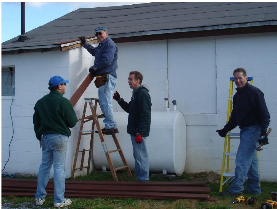
Club members, including Dale Litwhiler and Rick Lauter (both to right) repair the clubhouse roof.
